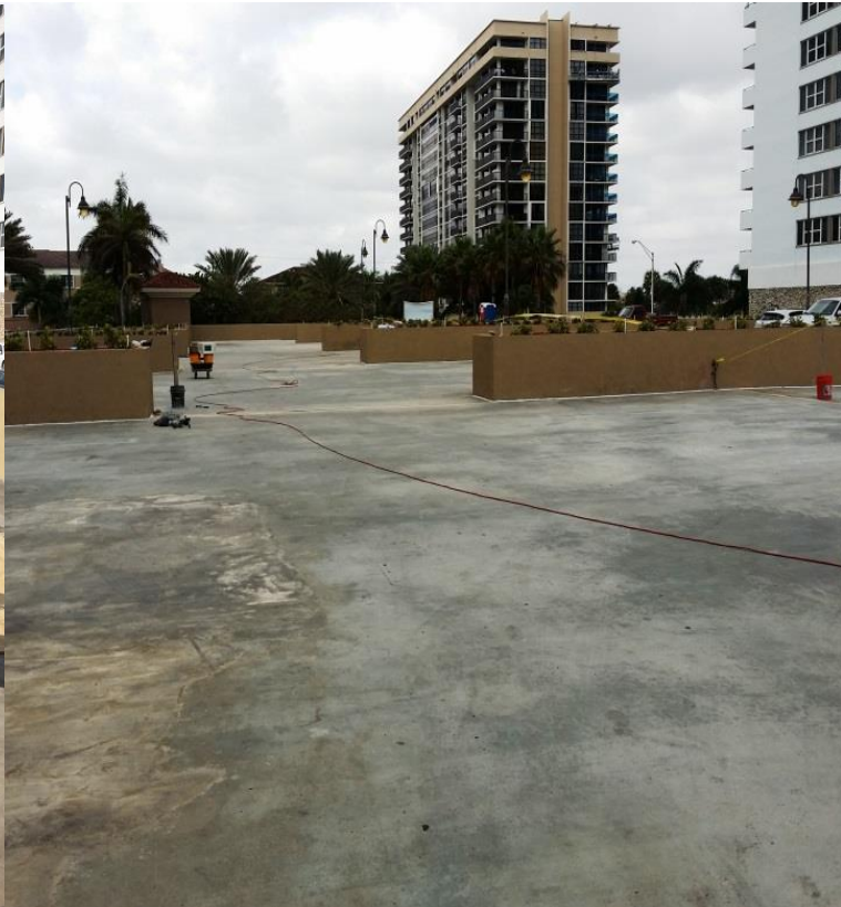
Existing Deck Condition
